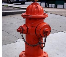
Gambar 4. 32 Hydrant outdoor (Sumber: verticalblinds.co.id)
