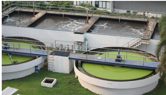
Gambar 10. Fasilitas Pengolahan Air Limbah (Wastewater Treatment Facility)
