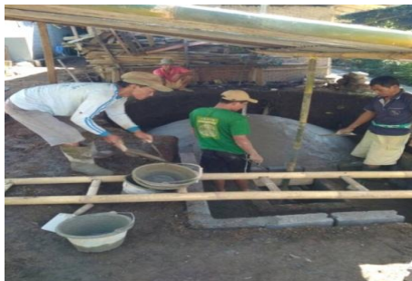
Gambar 3.5. Pilot project biogas
