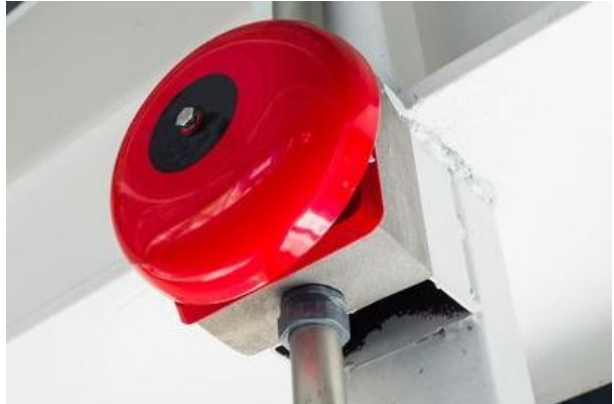
Gambar 4. 49 Fire Alarm (Sumber: www.pinterest.com )
