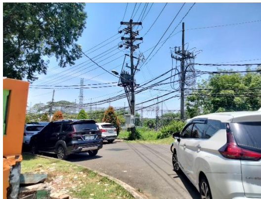
Gambar 4.15 Gardu Distribusi Listrik
