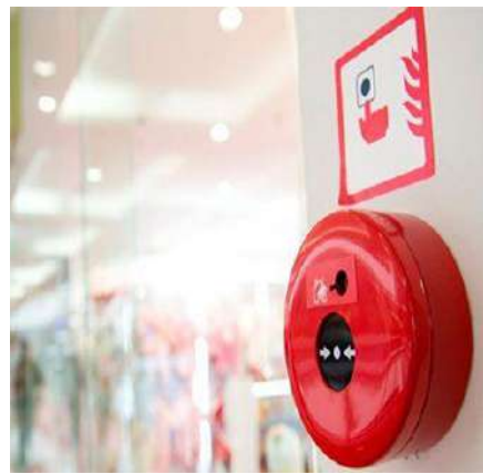
Gambar 5Gambar 33 Fire Alarm
